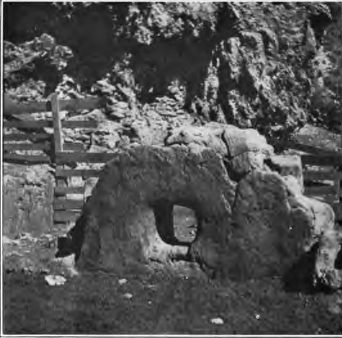
Remains of plastered walls
